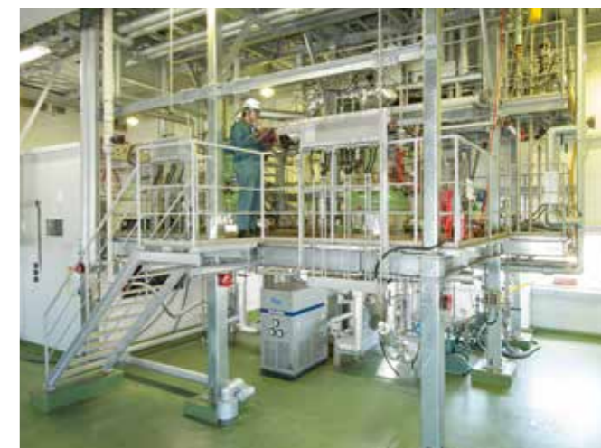
有機中実験設備 / Pilot Plant for Organic Iodine Compounds
