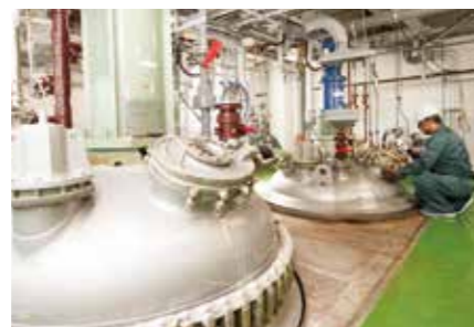
ヨウ素酸塩製造設備 Iodate Manufacturing Equipment
