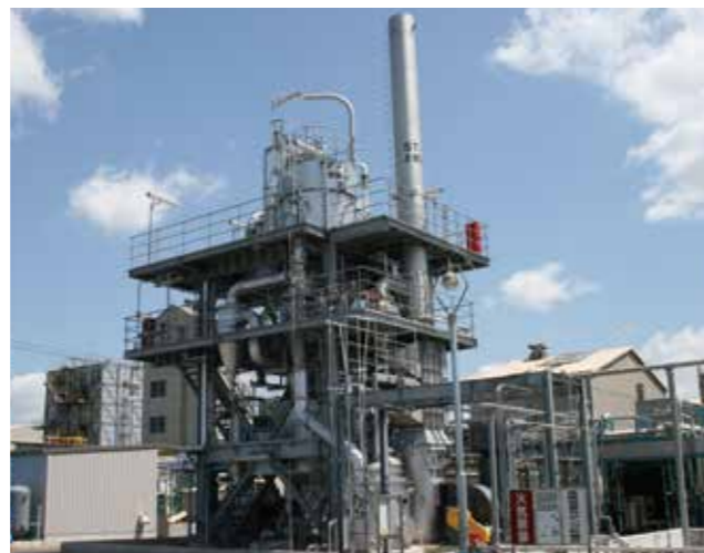
液中燃焼設備 / Submerged Combustion Equipment
