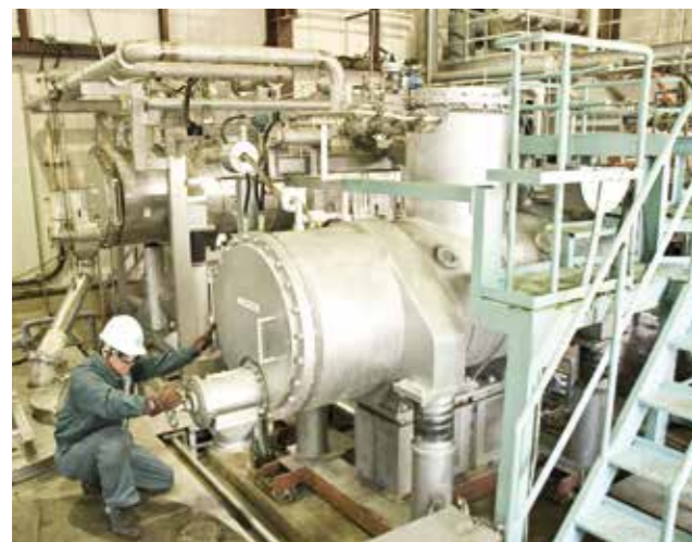
前処理設備 / Pretreatment Equipment
