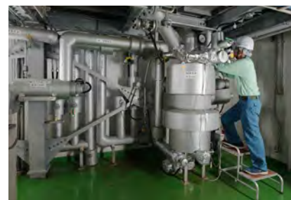
High-purity hydrogen iodide gas manufacturing facility
